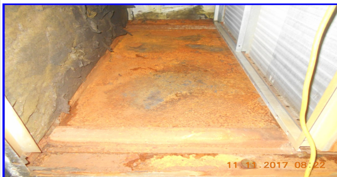
AHU DRAIN PAN BEFORE
