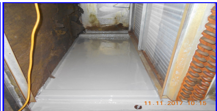
AHU DRAIN PAN AFTER
